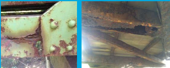
Rust Holes in Steel Members
